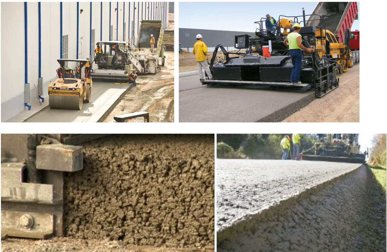
Figure 1. Construction of a road made of RCC and the appearance of the placed concrete
