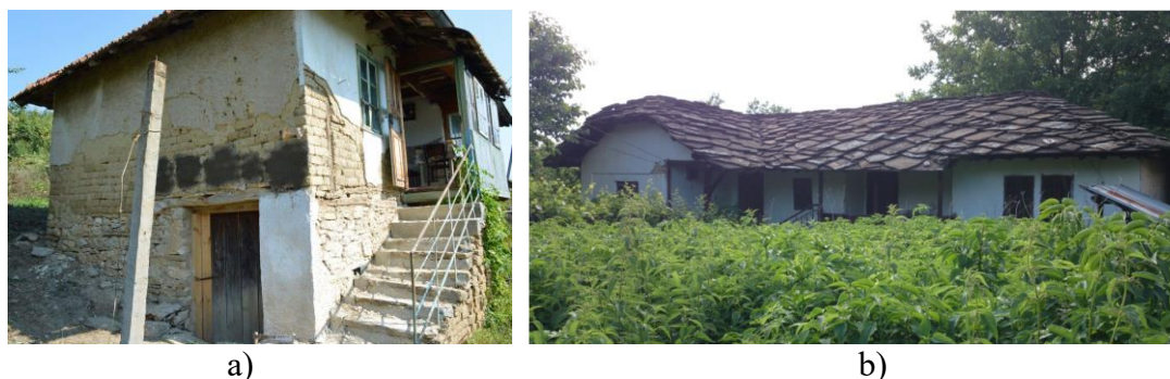
Fig. 6. Examples of negative practice: a) Bogdan Bogdanov house, Karpačevo, completely dilapidated; b) Christo Karpachev house [8]
