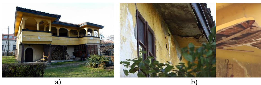
Fig. 2. Katić's house in Trstenik: a) Current condition of the building exterior; b) Visibly dilapidated façade and ceiling damage [16]
