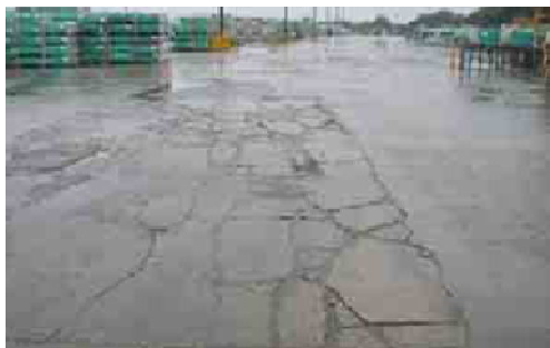
Figure 2. Condition of the driving surface
