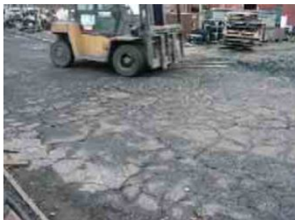
Figure 7. Condition of the driving surface
